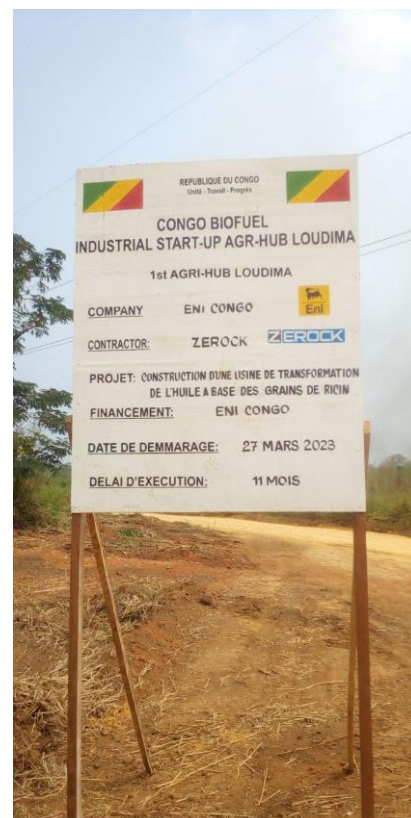
Sign at Eni's agri-hub construction site in Loudima, Republic of Congo. Photo: Marien Nzikou-Massala
