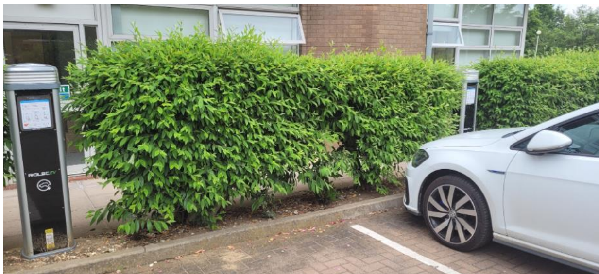
Figure 12: Workplace charging installed at Willmott Dixon's Hitchin office 12
