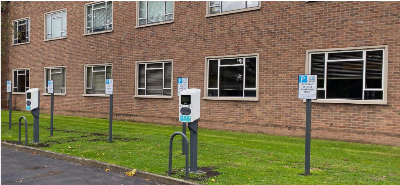
Figure 13: EA Technology Workplace Charging Installation 14
